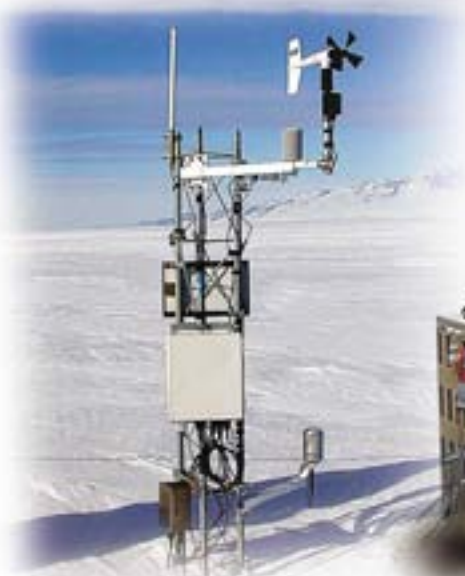
Outdoor weather station
